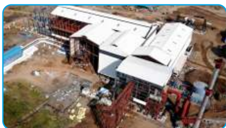
2000 TCD Boiler Capacity - 35 TPH 67 Kg 510 0 C Turbine : 6 Mw
